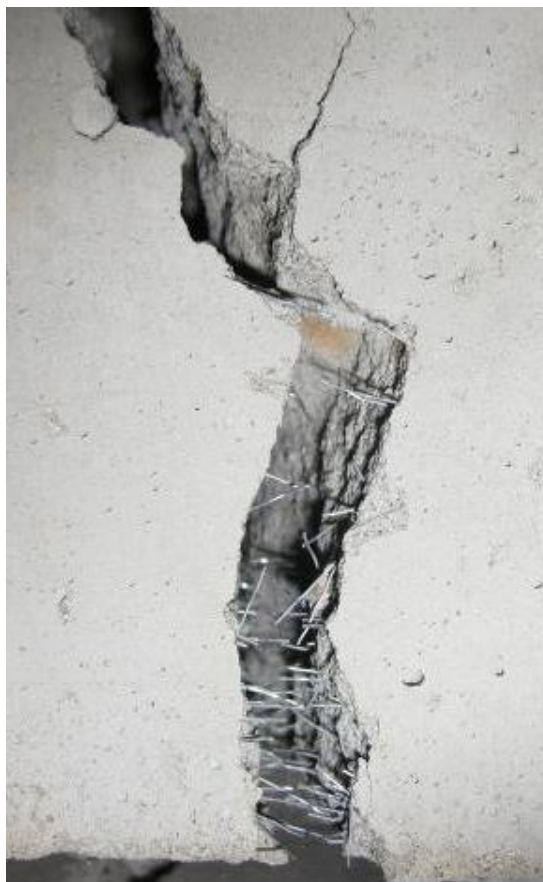
Fig. 4. Failure character latching
