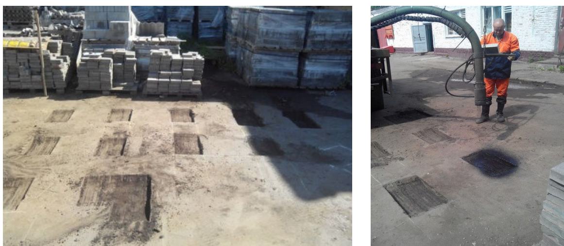
Fig. 3. Preparing areas of surfacing for laying a mix using the liquid-injection method and filling potholes with a bitumen mineral mix
