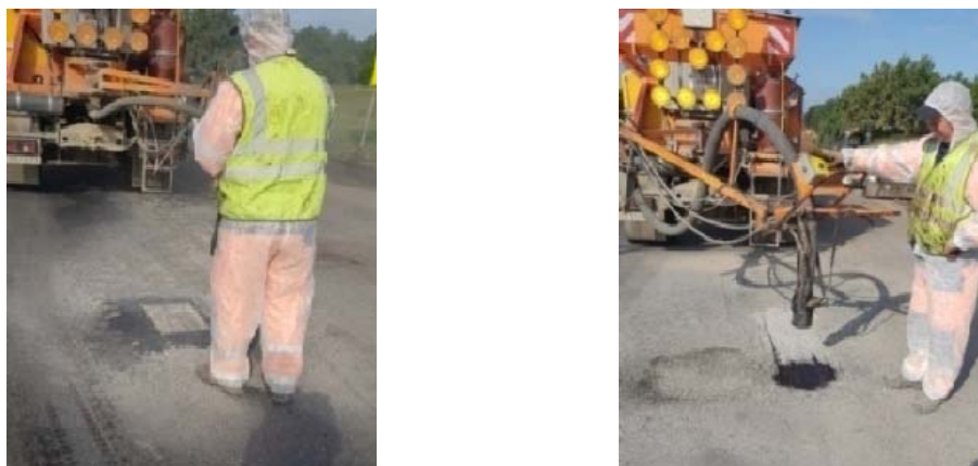
Fig. 2. Preparation of the area for the pothole repairs and filling it with the mix
