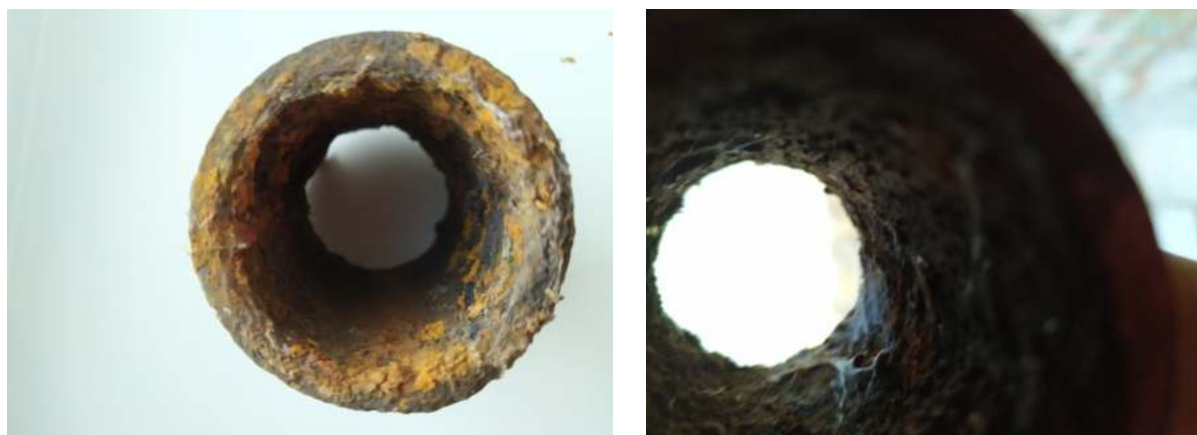
Fig. 2. A pipe with the diameter of 60 mm after 16 years of operation
