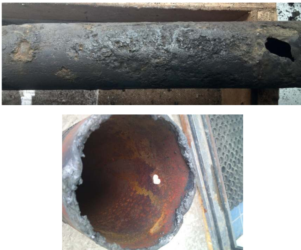
Fig. 1. Corrosion-damaged gas pipelines (photo by A. Yu. Chilikin)
